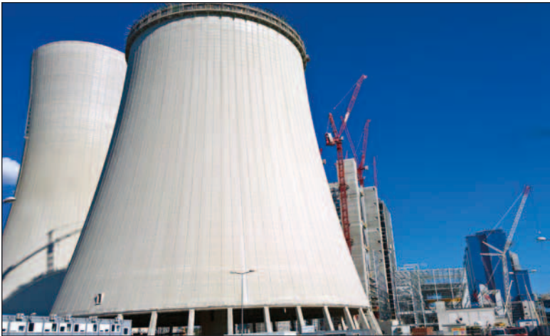
The expansion of the Opole Power Station, new cooling towers, photo by Konrad Górný, 2016
